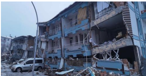
a) Soft storey irregularity-Column rupture (Kahramanmaraş)
