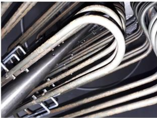
Figure 10: Inside view of the innovative steam peeling system (steam distribution pipe and resistances).
