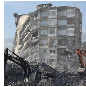
c) Torsional and soft storey irregularities (Gaziantep)
