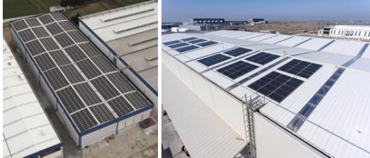
Figure 7: Solar Energy Systems Mounted at Roof Level [15,16]
