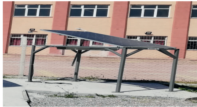
Figure 1: Fixed PV panel
