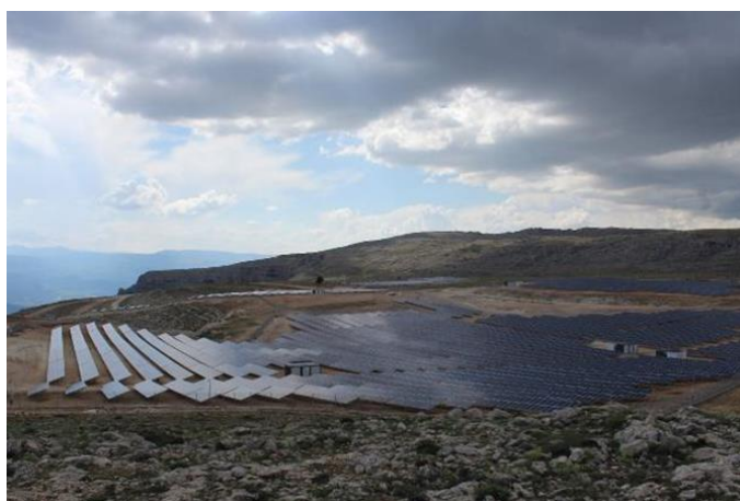
Figure 3. Ermenek Power Plant
